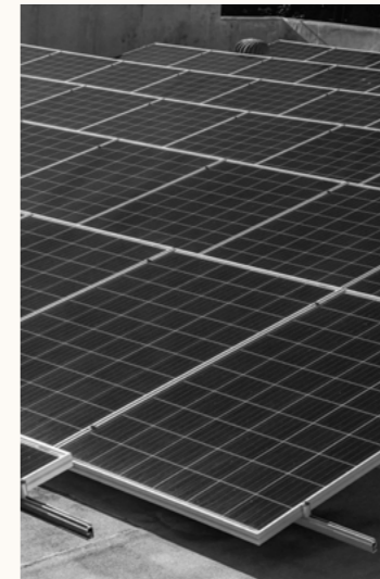
▲ Solar panel installations
